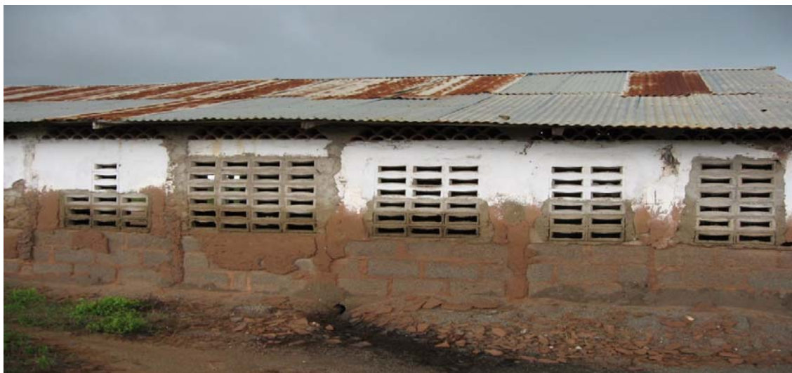
Fig. 7: Debilitative effects of salinity observed on wet salting curing premises structures at Maraikani, Coast province in Kenya. (Photograph by Mwinyihija)
